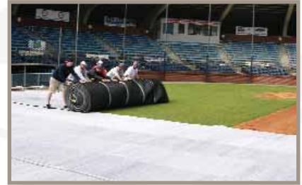
The 16' x 150' strips of EnkamatPlus are simply rolled out onto the field and held in place with ordinary landscape staples. Total installation time was less than 3 hours.
